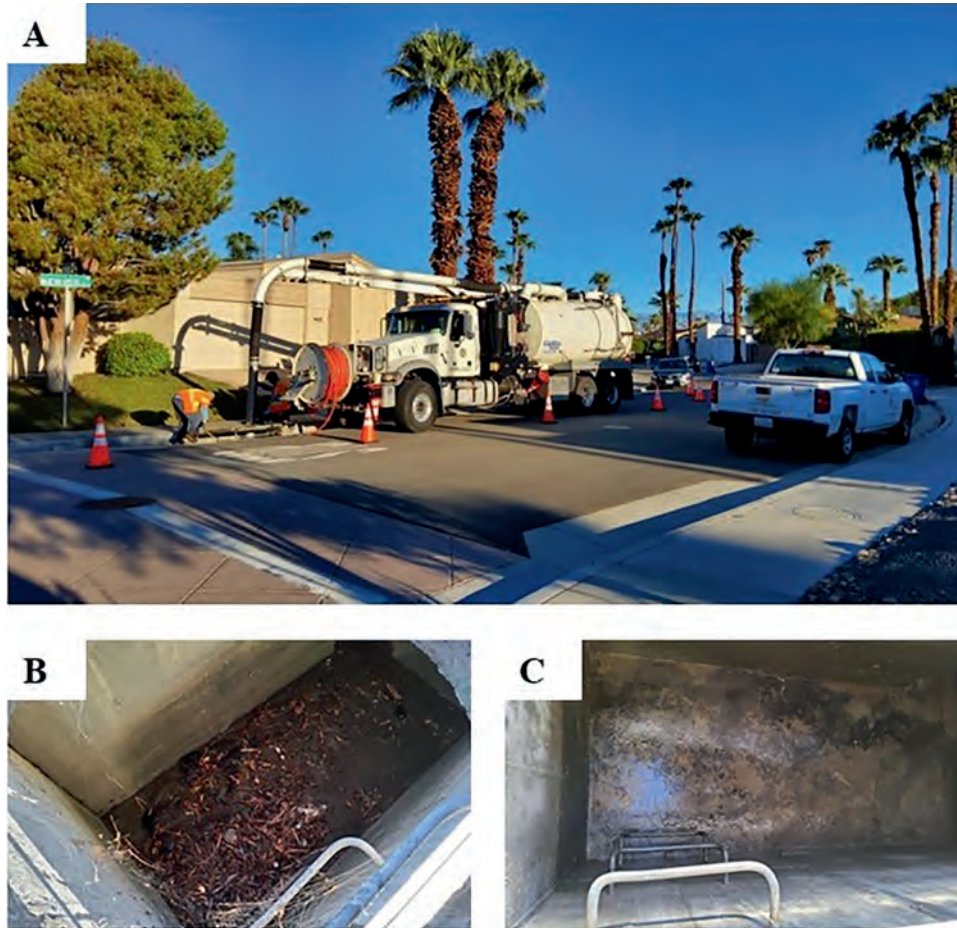
Figure 1. —Example of a catch basin clean out in Palm Springs. A) Veolia North America, a contracted group, cleaning out a catch basin in the city of Palm Springs using a GapVax truck. Water is used in conjunction with the built-in vacuum to clean out the drains. B) Catch basin site before cleaning. C) Catch basin site after cleaning.
