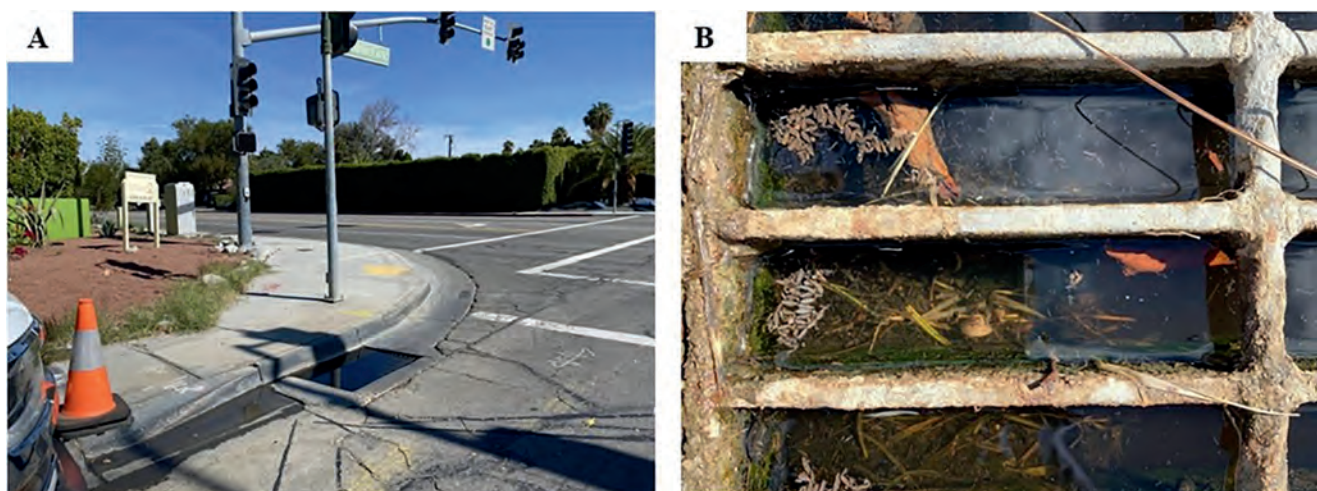
Figure 2.—A) Siphon drain at an intersection in Palm Springs. B) Egg rafts and mosquito larvae inside the drain.
