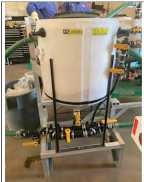
Figure 3. —Venturi equipment used for mixing the control product.
